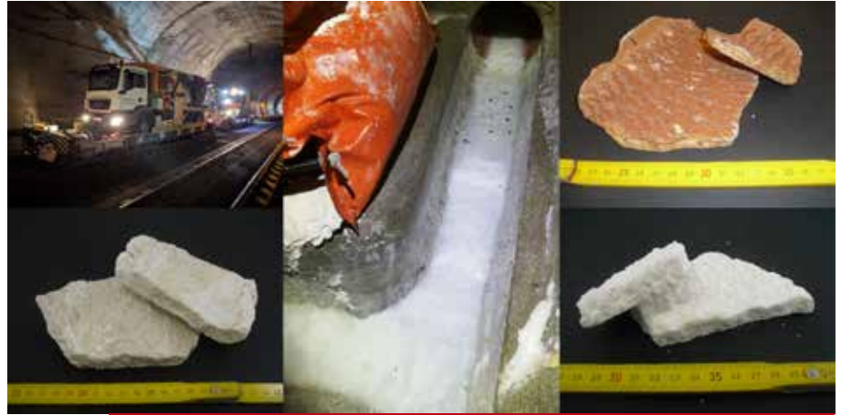
Drainage-Reinigung mittels Hochdruckspülung und unterschiedliche Ablagerungen aus Tunnel drainagen [2] Drainage cleaning by means of high-pressure flushing and different deposits from tunnel drainage [2].
